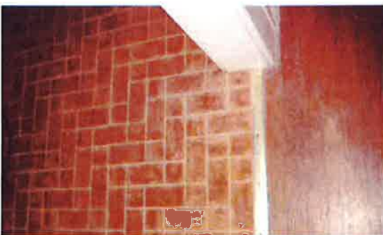
3 - Vinyl Flooring in Kitchen - to be removed and wood floor restored if possible
