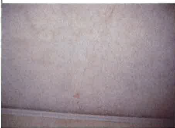
9 - Damage to Plaster Ceilings - to be repaired
