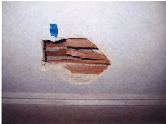
8 - Damage to Plaster Walls - to be repaired
