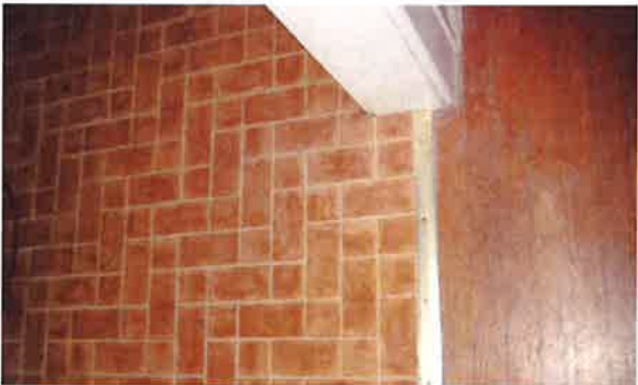
3 - Vinyl Flooring in Kitchen - to be removed and wood floor restored if possible
