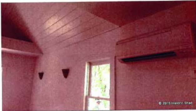
A mini split AC system provides heat and cooling
