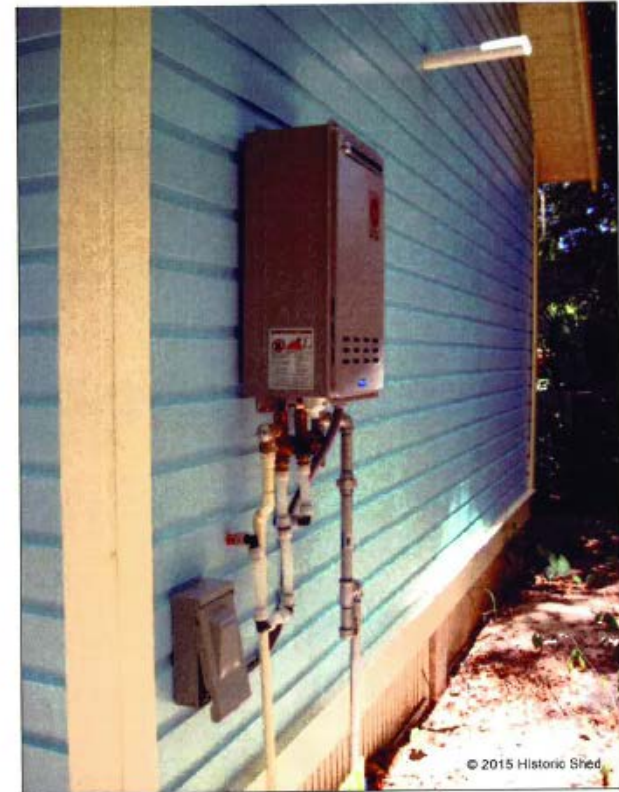
A gas tankless heater is located on the rear of the building
