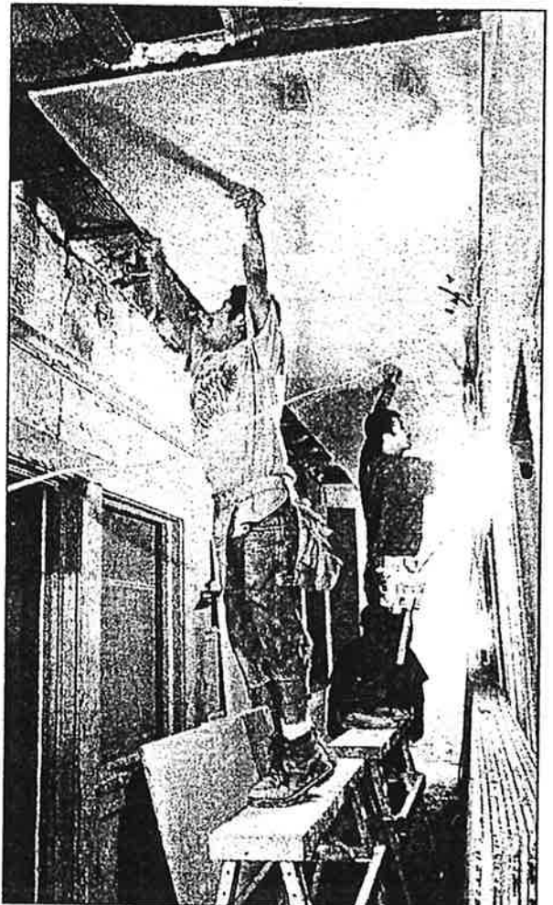
Gonzalo Hernandez (left) and Pedro Mendez work to renovate the W.A. Knight Building on West Adams Street. The project received city incentives. — Will Dickey/staff
