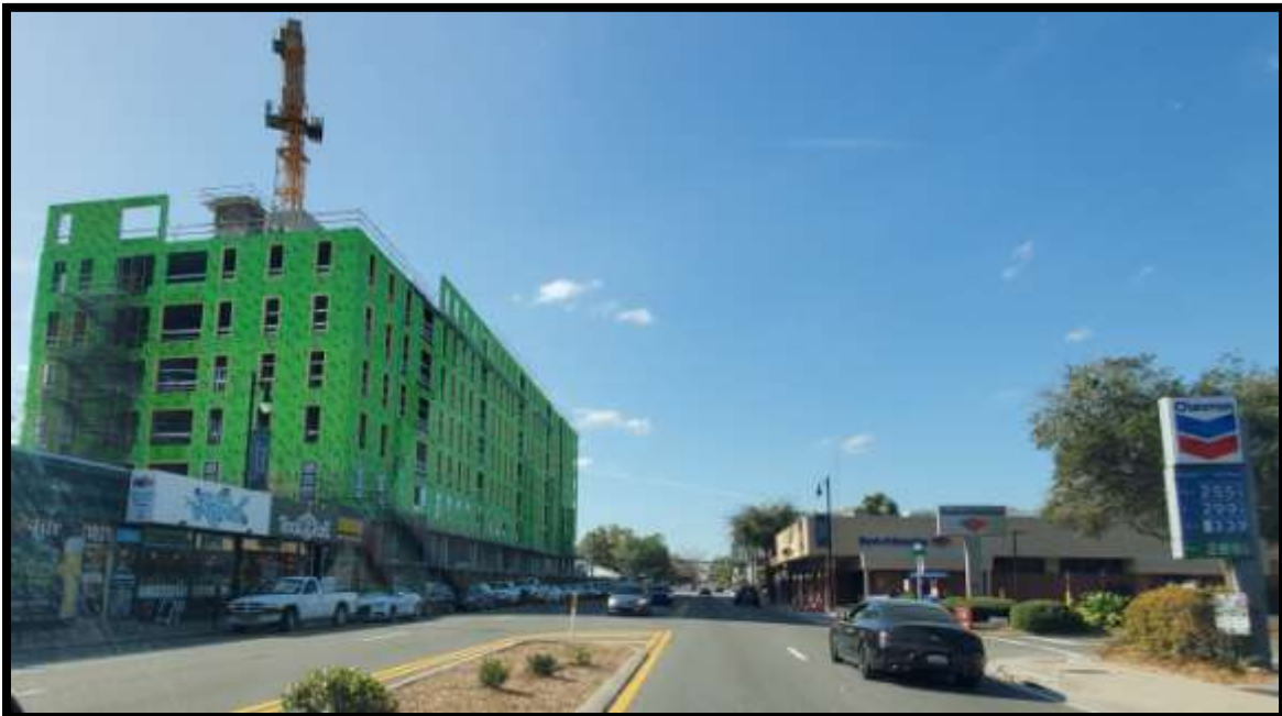
Under construction, the eastern portion is Sale #5 and the western portion is Sale #4
