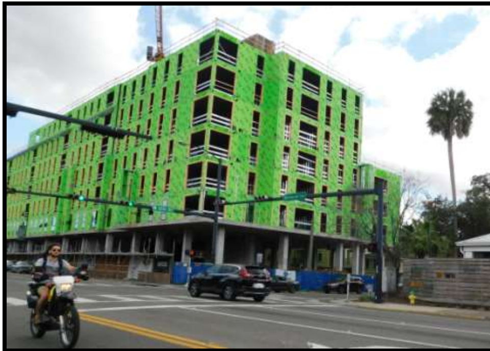
Currently under construction, the western end of the development covers this sale.
