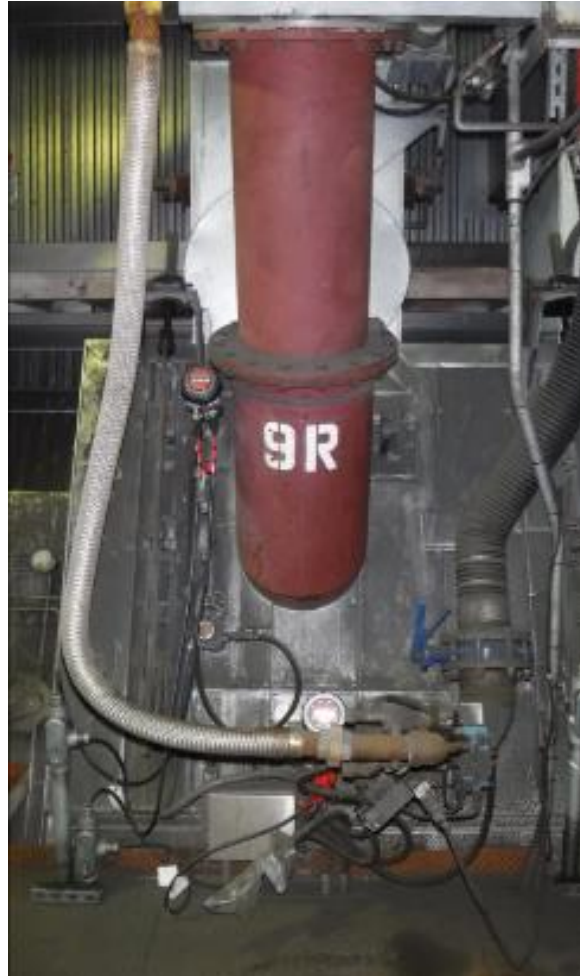
Existing Coal Pipe Elbow
