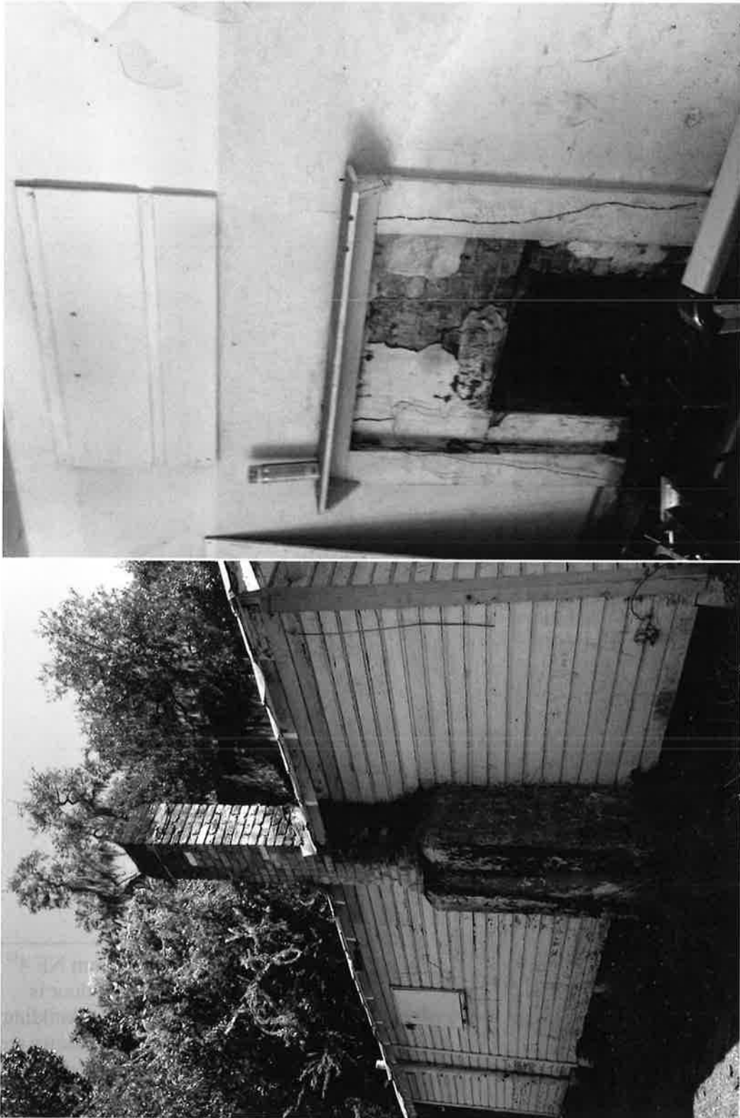
View of chimney from interior and exterior. The exterior of the chimney has minor mortar and brick damage and invasive vine growth. The interior wall appears to be in good condition.
