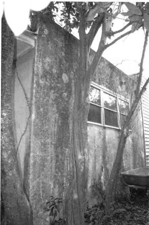
9 (top): Rear (west) elevation, showing rear porch addition on left and master bedroom addition on right. Note removal of roof parapet wall on this west elevation of master bedroom addition.
