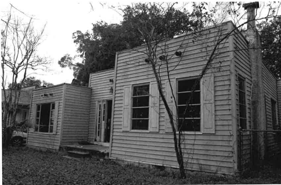
4: North elevation of original carport, where smaller arched opening has been covered with siding. Original stucco chimney visible on the right (north elevation).
