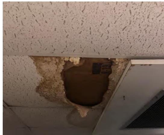
Figure: Stained and damaged ceiling tile in the second floor bunk area.
