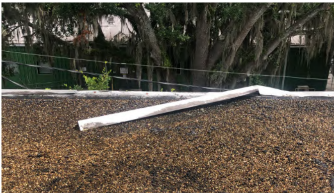
Figure: Damaged eave flashing as seen from the second floor roof.
