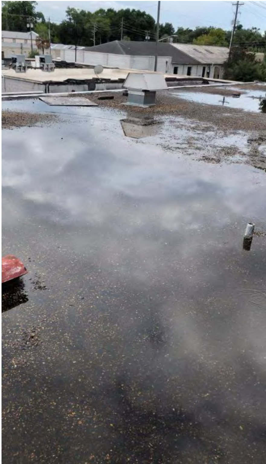
IMAGE 8: STANDING WATER ON ROOF OVER APPARATUS BAY
