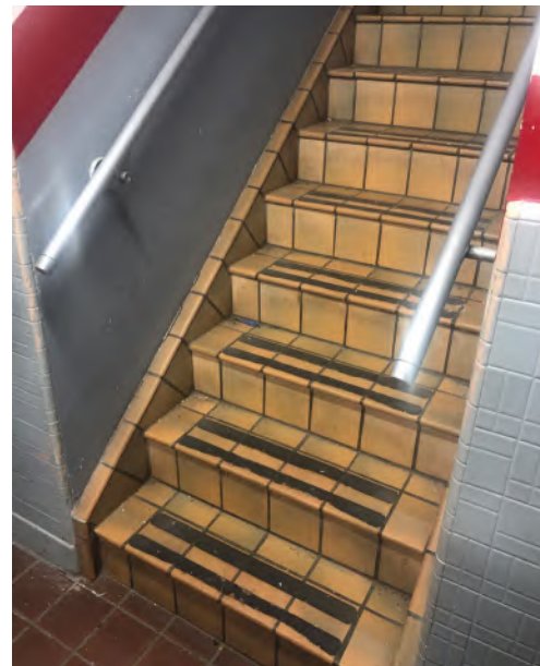
Figure: Stair leading up to the second floor. Built at 39" wall-to-wall with 2" wide handrails.
