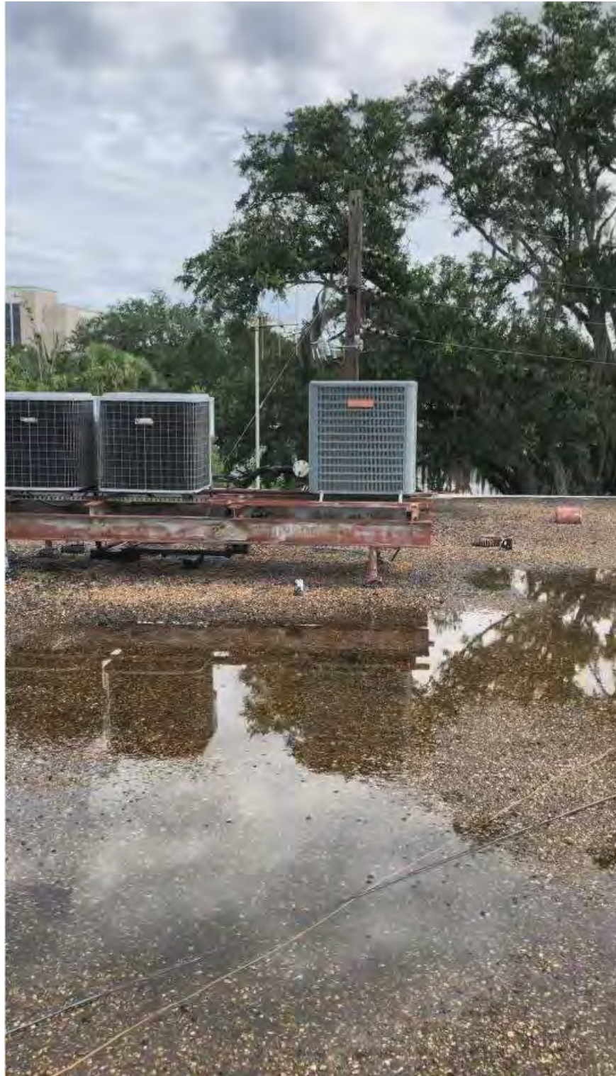
IMAGE 9: STANDING WATER ON ROOF OVER TWO-STORY SPACE
