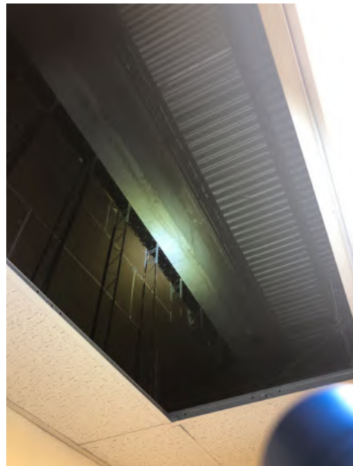
Figure: Removed ceiling panel reveals the masonry wall system with steel structural members.
