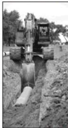
Construction workers install the city's effluent line near Harry McAdams Park in May 2016.
