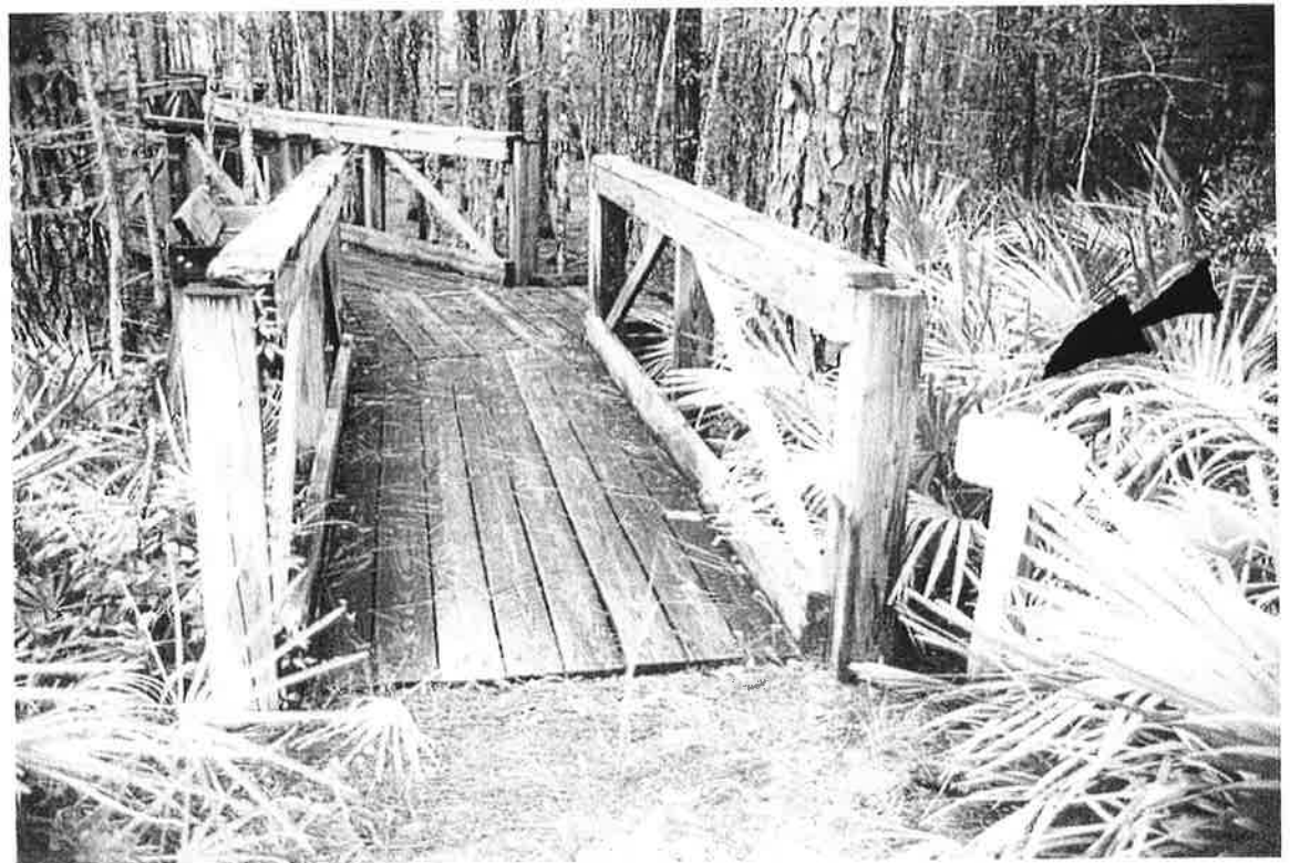
TYPICAL VIEW OF CYPRESS DOME BOARDWALK. NOTE "SLIPPERY WHEN WET" SIGN DUE TO MOLD GROWTH.
