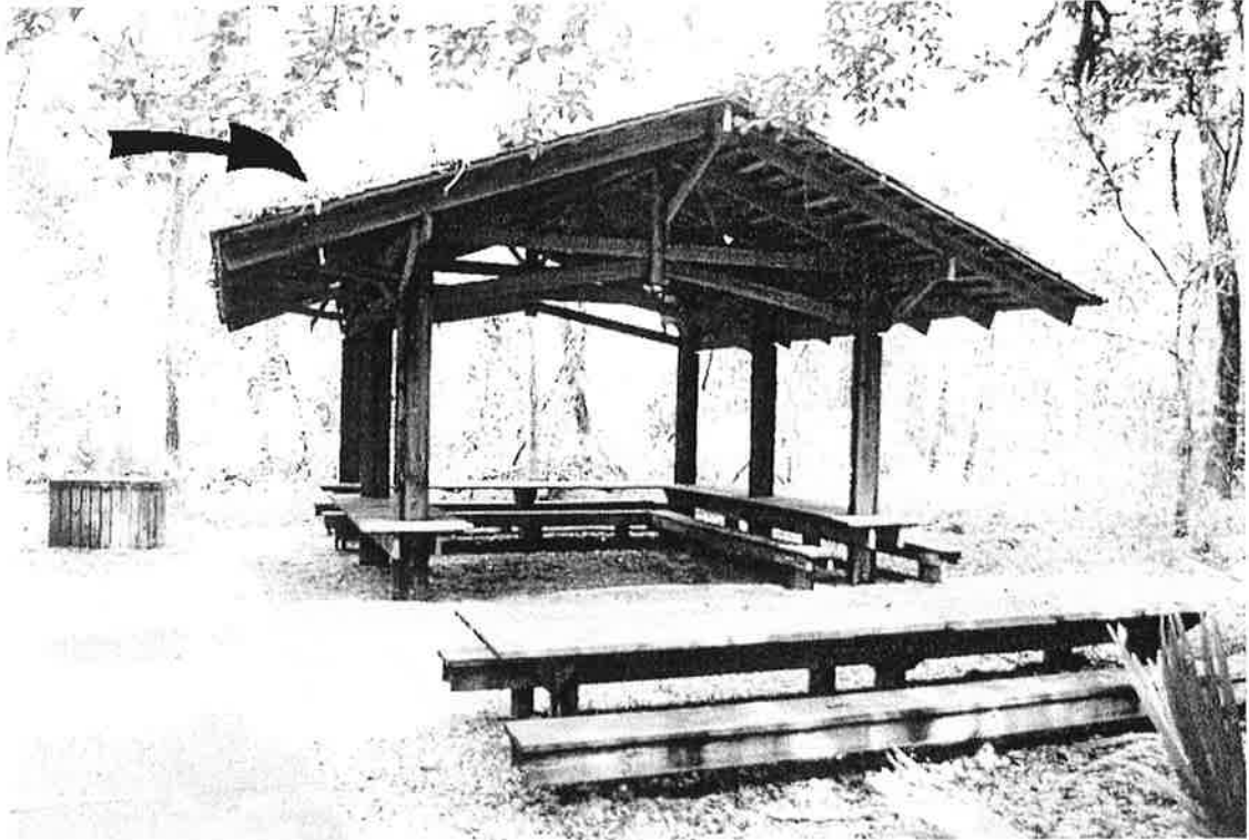
PAVILION - NOTE GROWTH ON ROOF AND MINOR DECAY WHERE THE POSTS MEET THE GROUND
