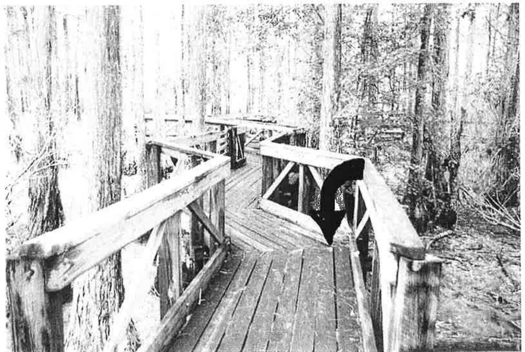
TYPICAL BOARDWALK VIEW. NOTE TWISTING AND WARPING OF DECKING.
