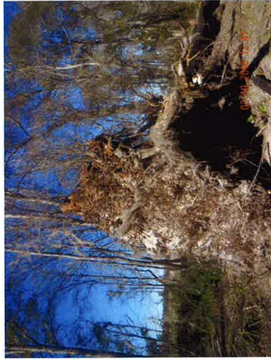
Examples of tree fall showing extent of exposed roots and depth of roots.
