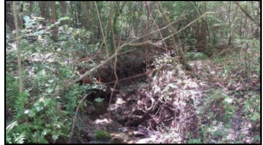
EXISTING ERODED AREAS IMMEDIATELY DOWNSTREAM
