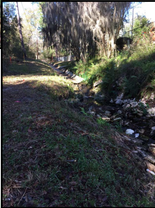
EXISTING ERODED AREAS IN PROJECT LIMITS
