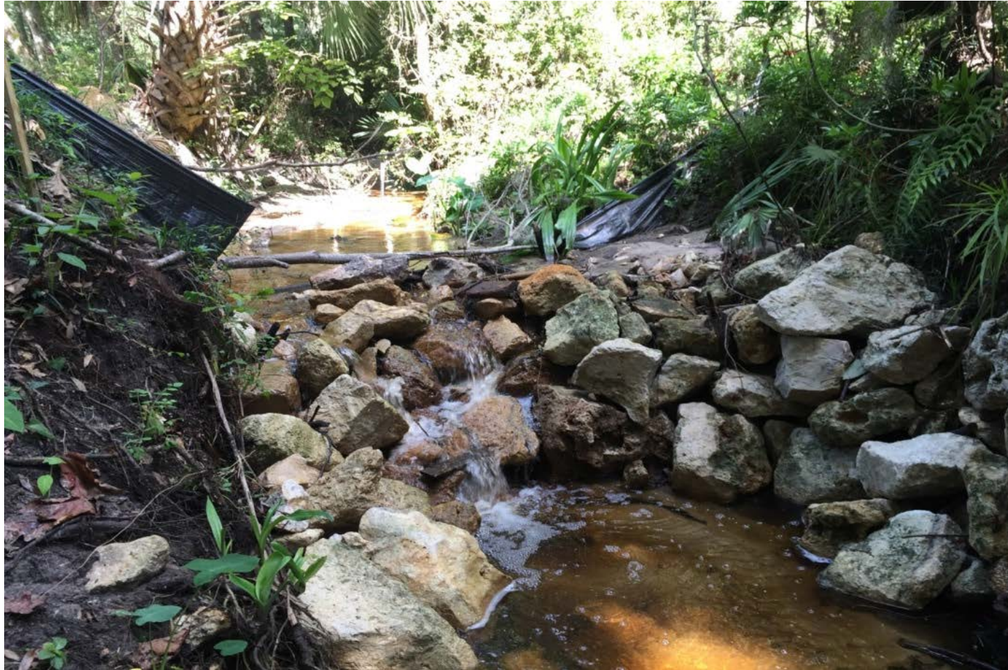
Beville Creek in Cofrin Nature Park during construction (8/19/2015). Large boulders creating a check dam for grade control within Beville Creek.
