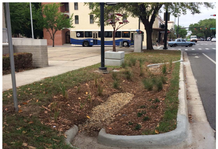
At our current streetscape project on South Main, we are installing low impact development stormwater facilities and associated landscaping.
