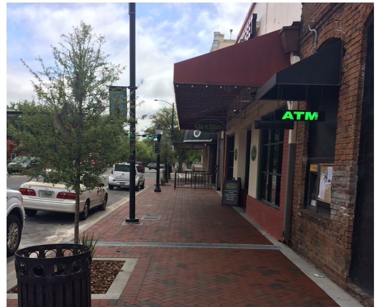
Our progress at South Main Street, under project manager Derek Dykes, involves removing and replacing trees, modifying ADA ramps and sidewalk slopes, and adding bus stops and rest areas with new benches.
