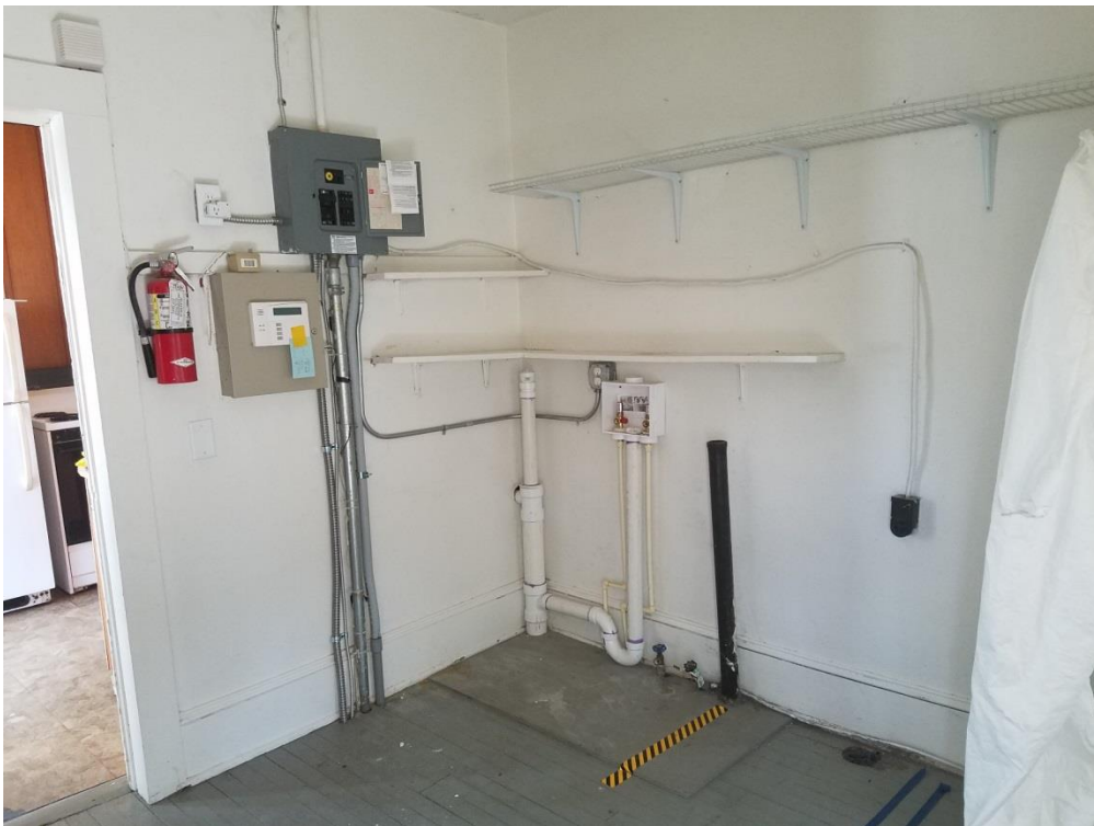
Utility room: view of rear wall (top) and view towards kitchen (bottom)
