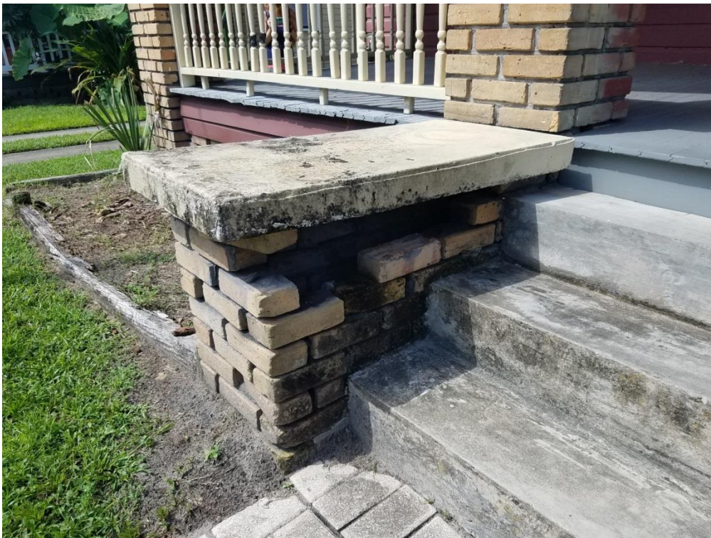
Examples of existing masonry piers and step hip wall which need to be repointed and rebuilt
