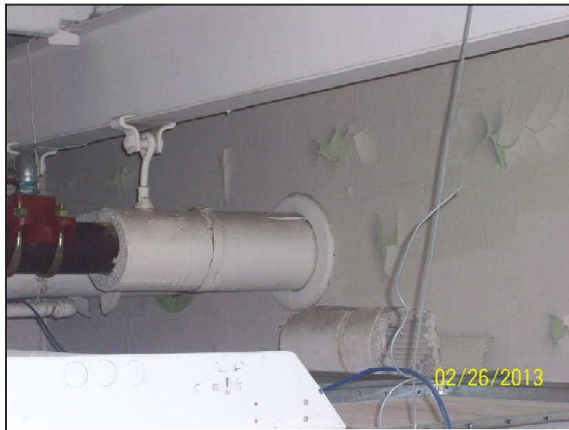
Photo 9: Confirmed ACM: pipe insulation (please note dislodged section)
