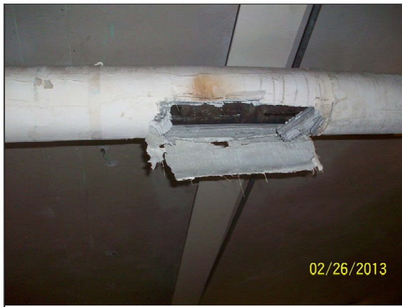
Photo 10: Confirmed ACM: pipe insulation. (Please note damage)
