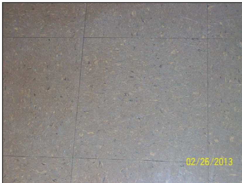
Photo 7: Confirmed ACM: mastic underneath 12-inch by 12-inch tan floor tile
