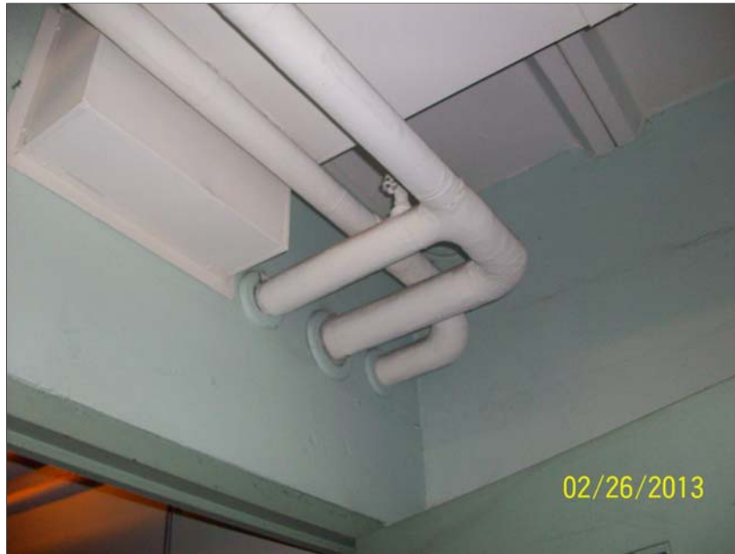
Photo 11: Confirmed ACM: pipe fitting insulation
