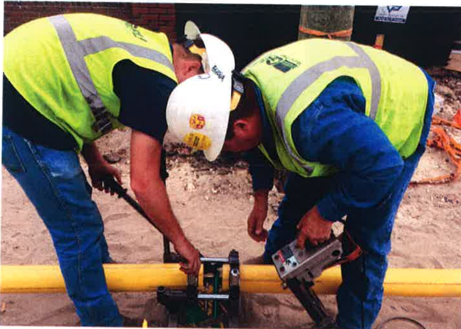
Crews sealing a HPDE gas line. These lines are compressed to make one long pipe to cover the length of the street.
