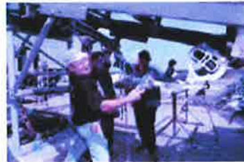
Dave Kranzler, left, Jeff Blayz and Randy Parvu work on a conveyer belt at Ajax Paving Industries early Wednesday. An official says it cost about $500,000 to fix the plant and put in some planned upgrades.
