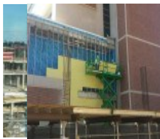
Panels are removed to allow the new hospitals to connect to the UF Health Shands Cancer Hospital.
