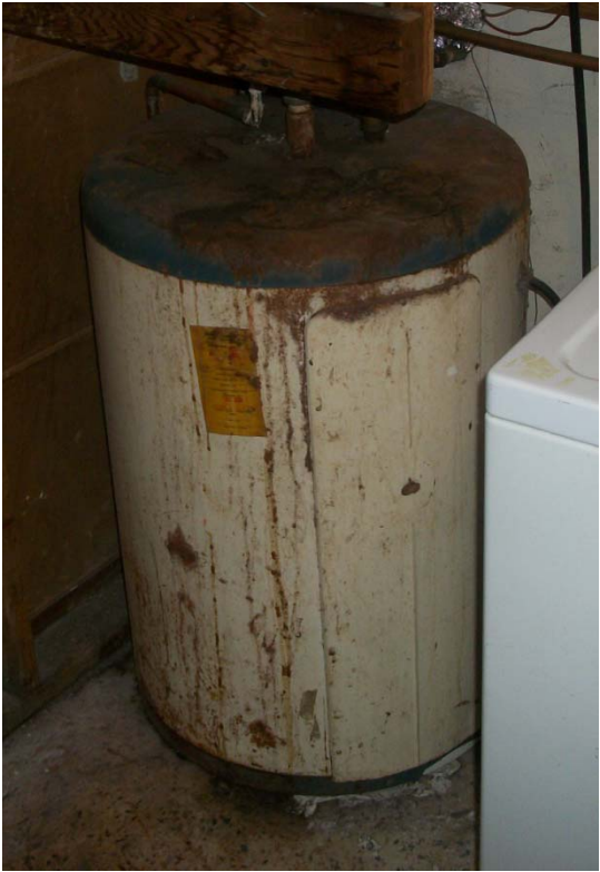
Water heater BEFORE
