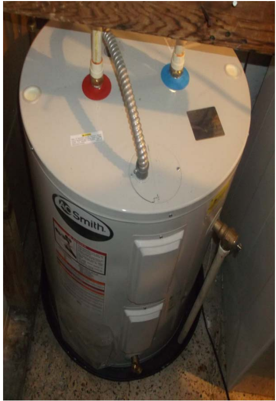
Water heater AFTER
