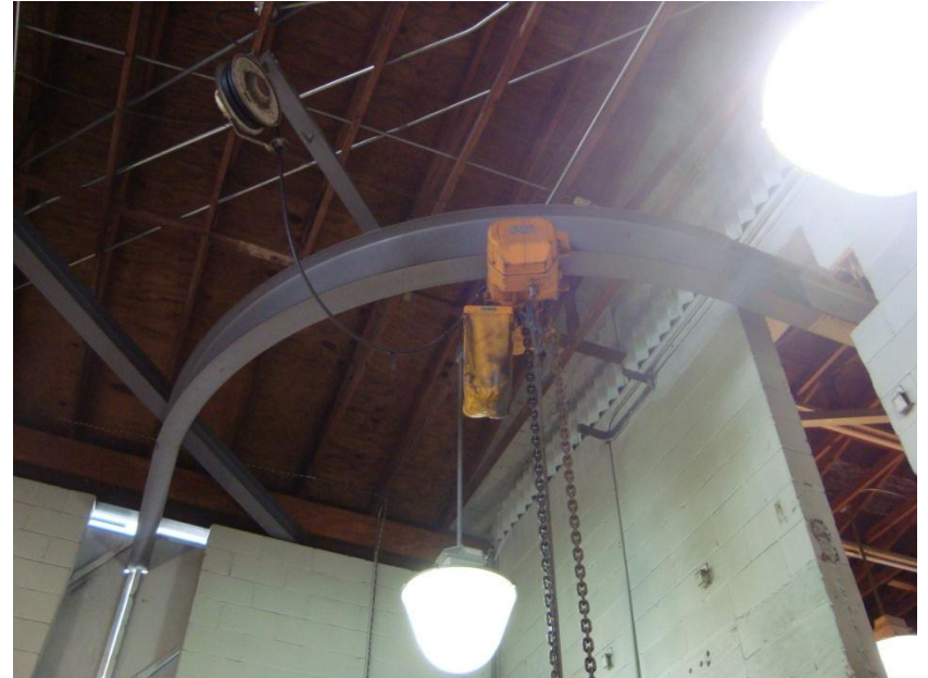
Ceiling Machinery Track
