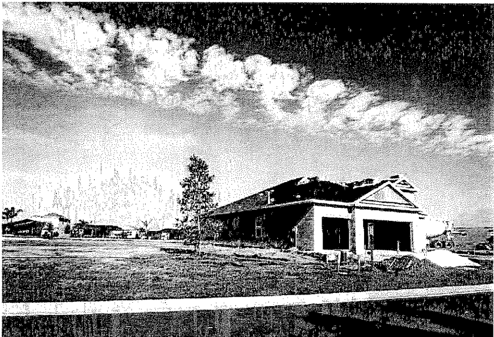
Work continues on homes currently under construction in Lakewood Ranch on Dec. 16.
