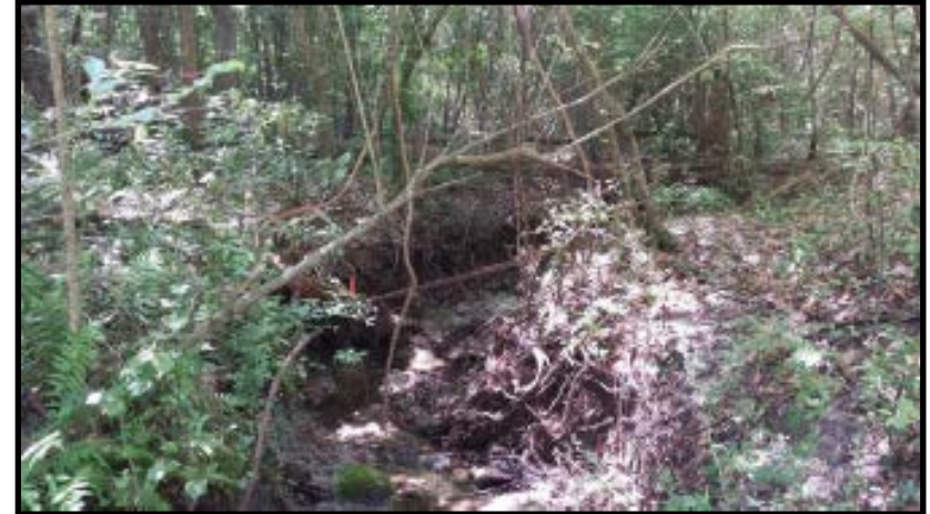
EXISTING ERODED AREAS IMMEDIATELY DOWNSTREAM
