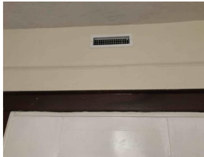
New AC vent in parlor
