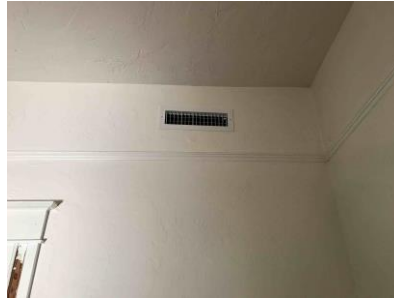
New AC vent in living room
