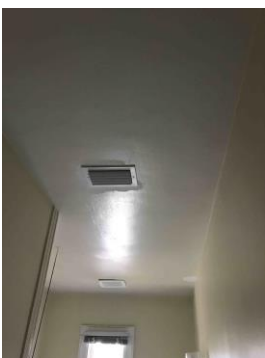
Upstairs east bath AC vent
