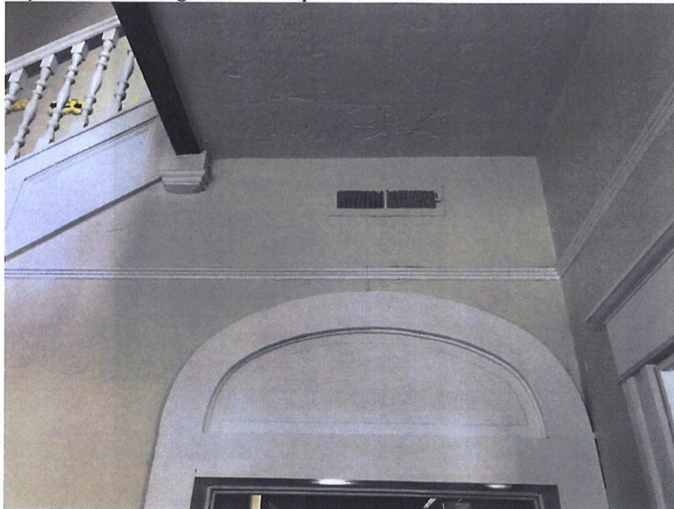
Foyer – New AC register will be placed at same location as old forced air vent
