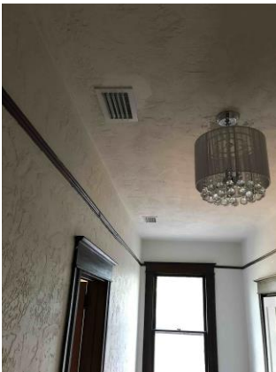
Upstairs hall AC vent
