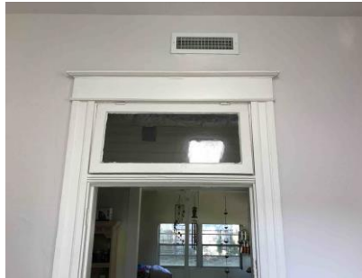
New AC vent in kitchen
