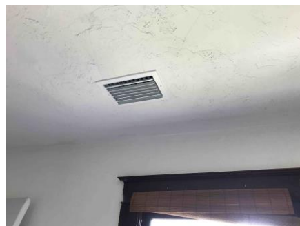
Upstairs north bedroom AC vent
