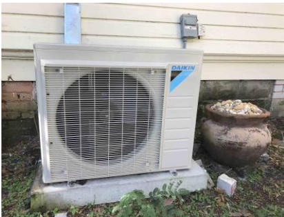
Mini-split outside unit
