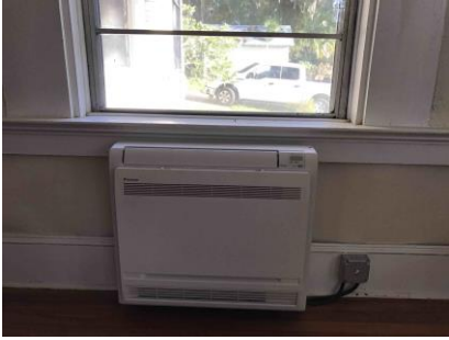
New Mini-Split in Sun Room
