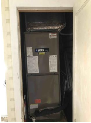
Downstairs air handler
