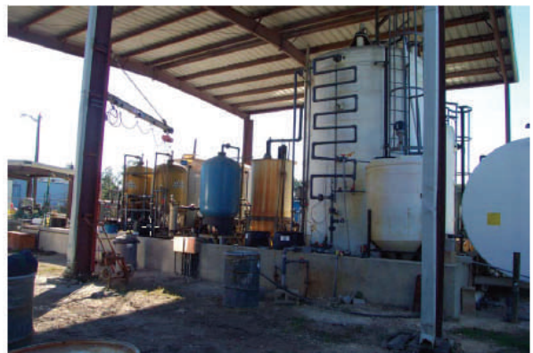
Water Treatment Plant, Interior View, Koppers
