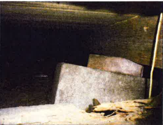
PHOTO 5 FOUNDATION SKEWED AND STRAPS MISSING
