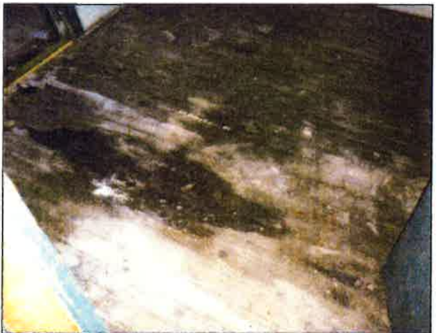
PHOTO 6 FLOOR SHEATHING IN POOR CONDITION
