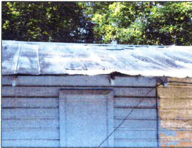
PHOTO 1 WARPED ROOF ROOFING REQUIRES REPLACEMENT
