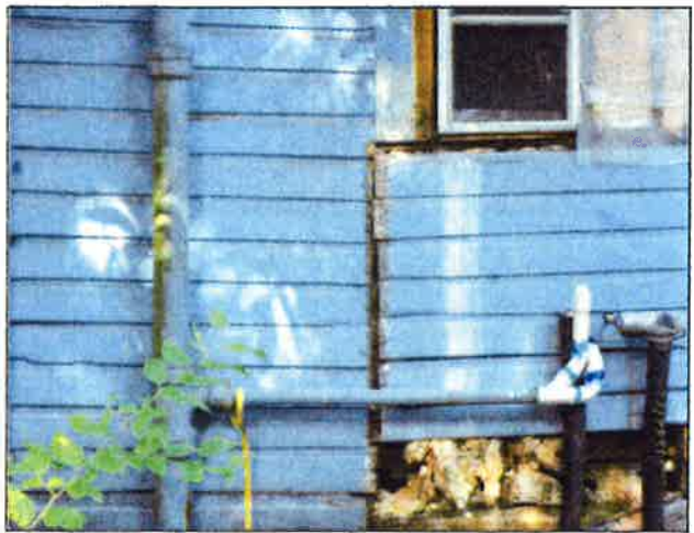
PHOTO 4 ROTTED WALL FRAMING AT BASE OF EXTERIOR WALL
