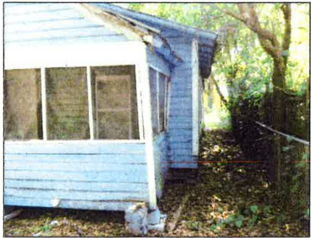
PHOTO 2 EXTERIOR BEARING WALL LEANING BEYOND STANDARD TOLERANCE
