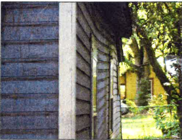
PHOTO 3 WALL SIDING OUT OF ALIGNMENT
