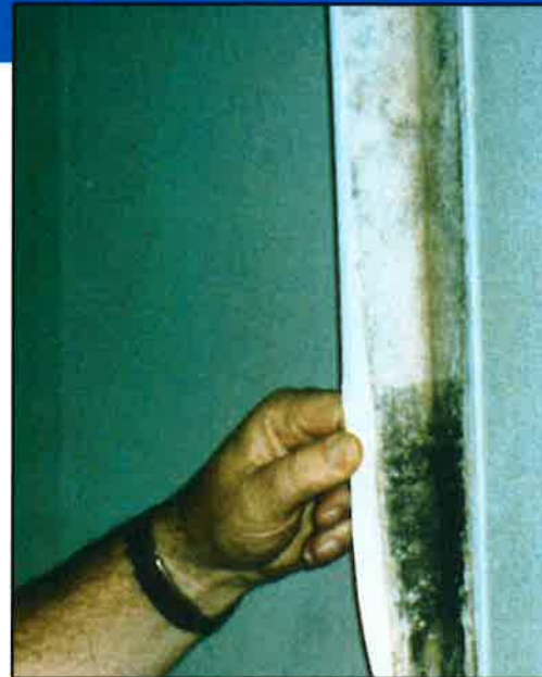
Mold growing on the back side of wallpaper.
