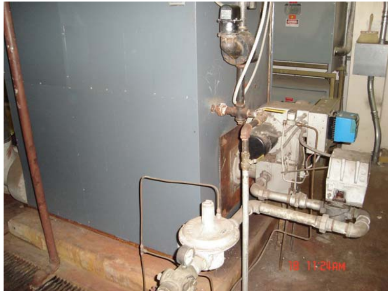
Existing Weil McLain Boiler
