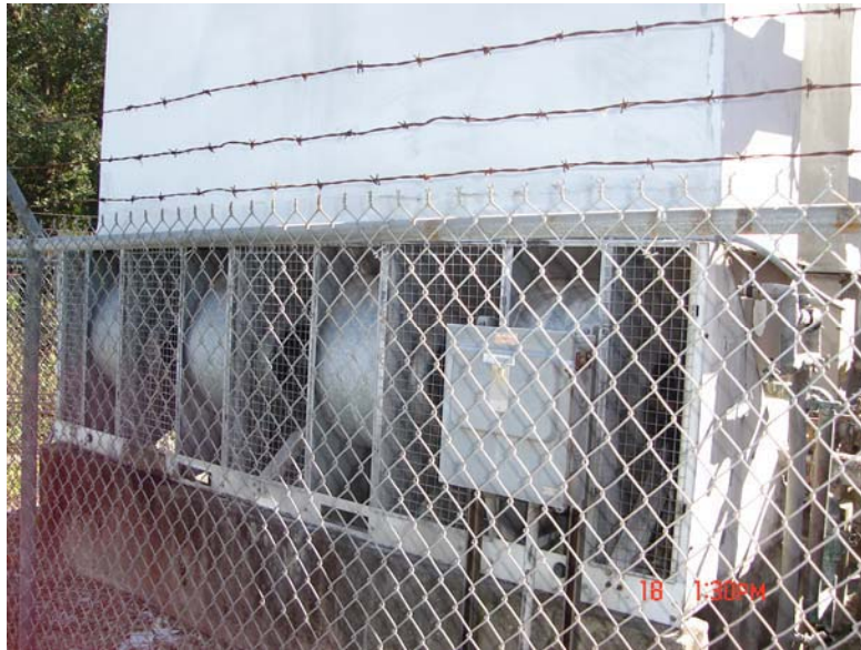
Existing Cooling Tower
