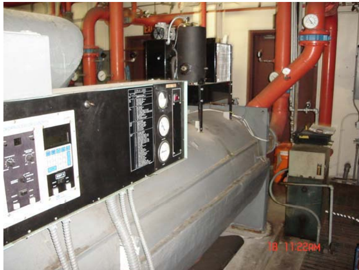
Existing Chiller at GPD
