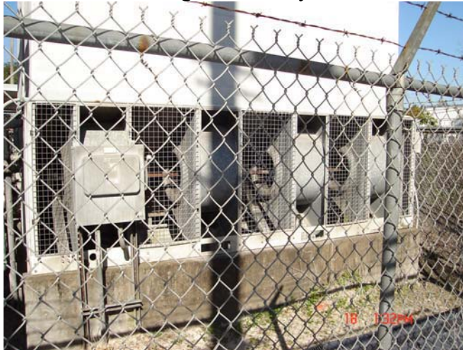
Existing Cooling Tower at GPD
