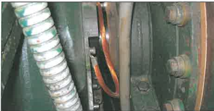
Unit 8 Generator Shaft Ground Device
