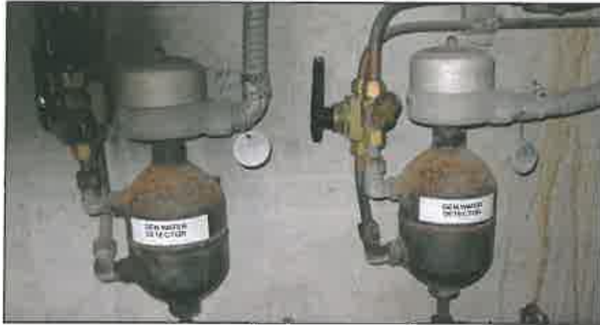
Liquid Level Detector showing valves for functional testing
