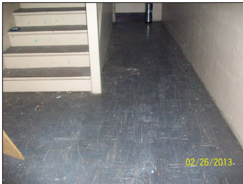
Photo 3: Confirmed ACM: 9-inch by 9-inch black floor tile and mastic
