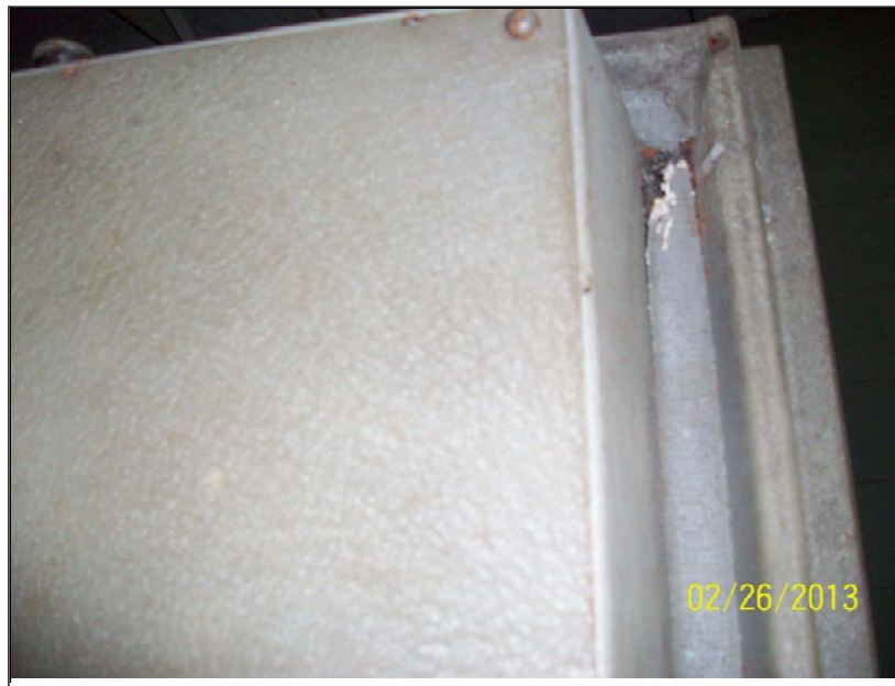
Photo 8: Confirmed ACM: woven gasket adhered to the seal of the arms vault door
