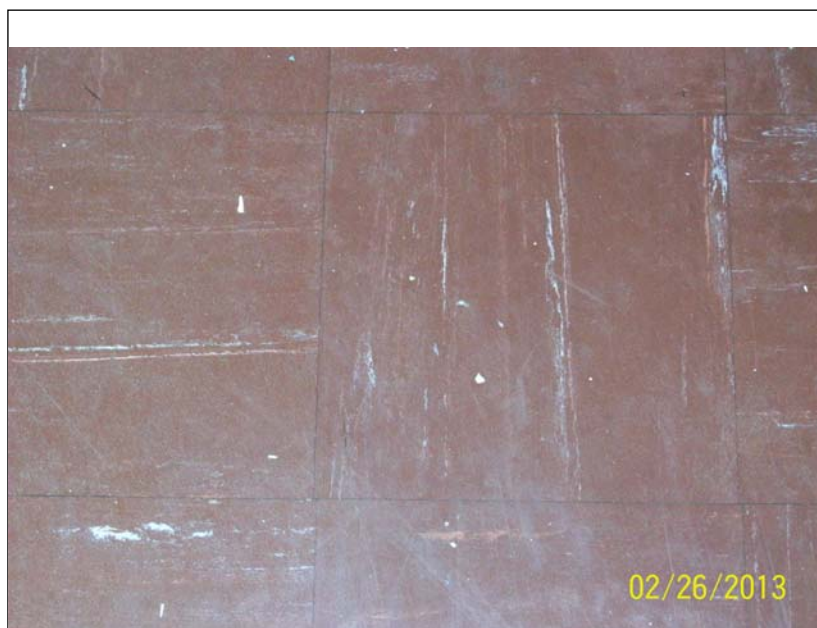
Photo 4: Confirmed ACM: 9-inch by 9-inch brown floor tile and mastic
