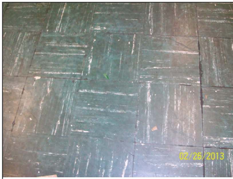
Photo 2: Confirmed ACM: 12-inch by 12-inch green floor tile and mastic
