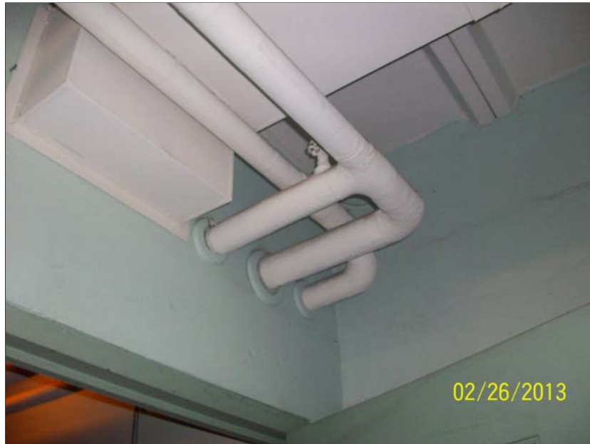
Photo 11: Confirmed ACM: pipe fitting insulation
