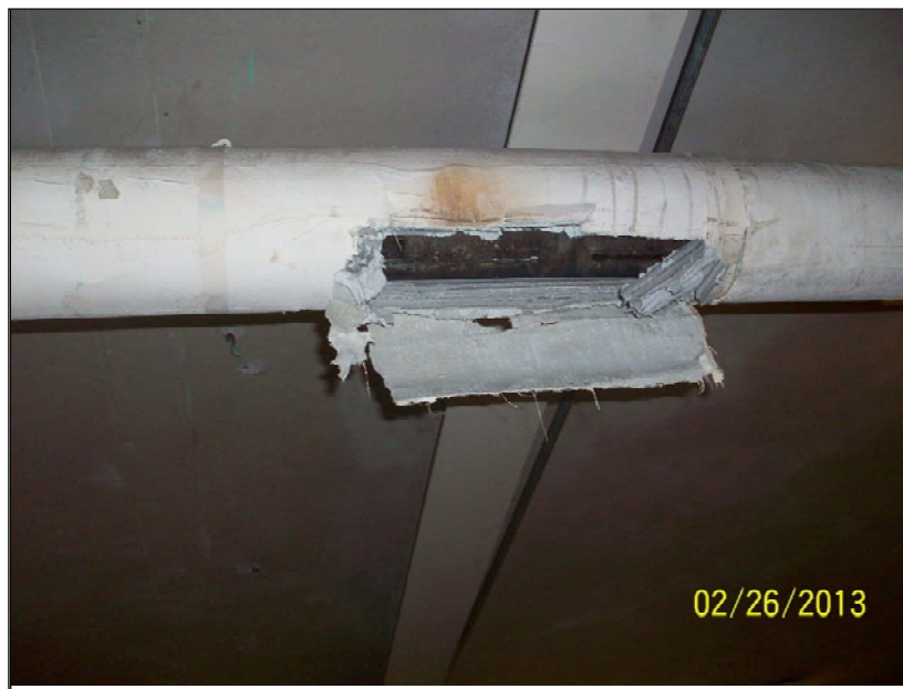
Photo 10: Confirmed ACM: pipe insulation. (Please note damage)
