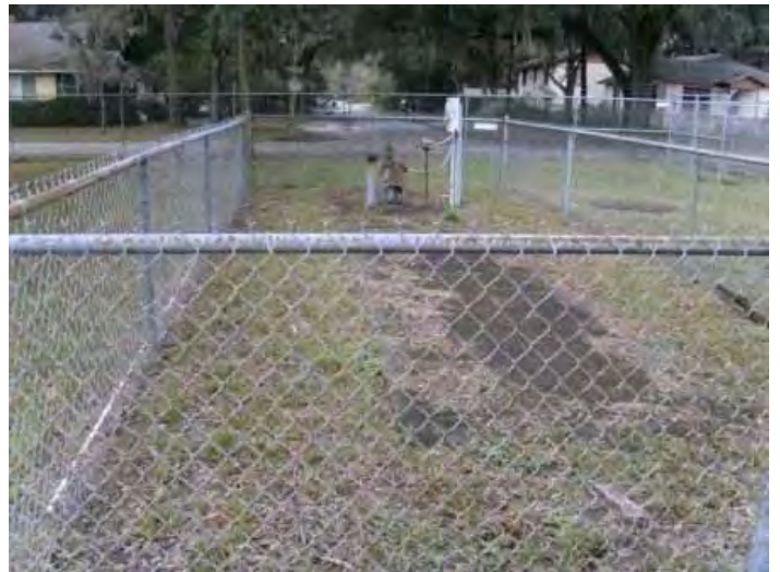
Oil Water Separator
