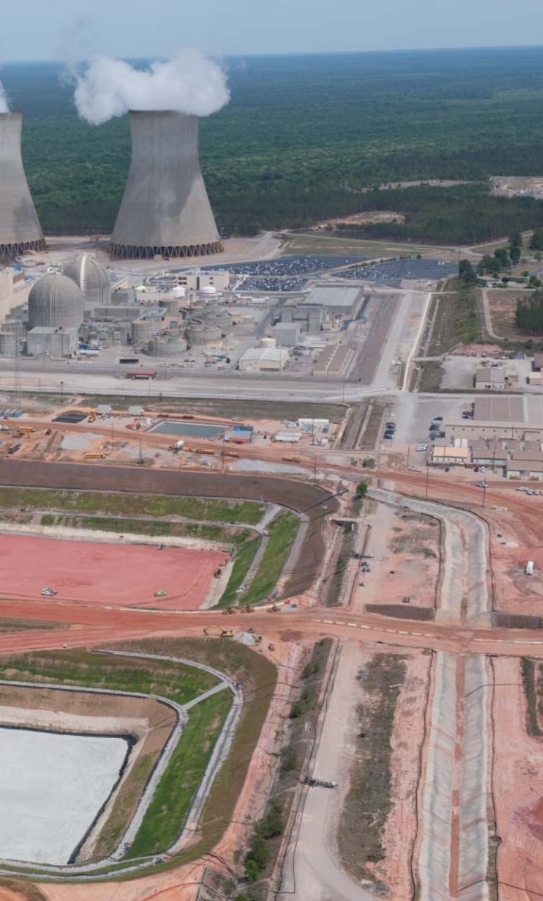
◀ Southern Company breaks new ground at the Vogtle site in Georgia, US
