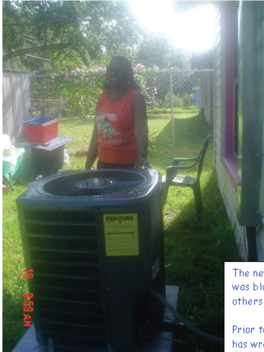
Gainesville resident, Brenda Stewart, standing by the heat & air conditioning unit that was installed in her home as part of the weatherization program to improve energy efficiency.
