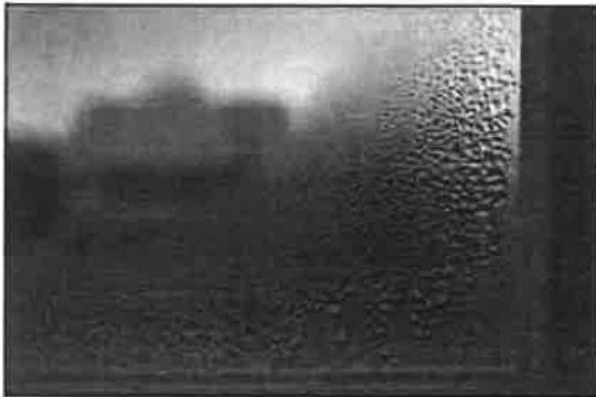
Condensation on the inside of a window-pane.
