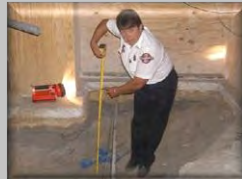
Fire Safety Inspections and Investigations
