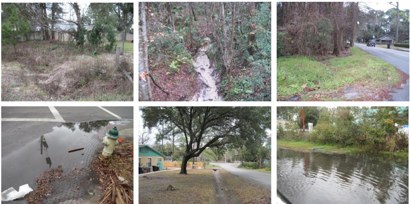
Figure 2-8: Examples of Inadequate Stormwater Facilities
