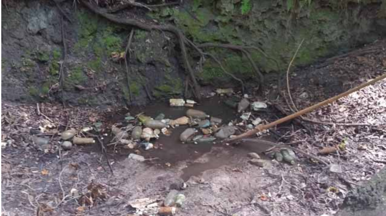
Figure 23. Standing water found in the bottom of one of the depression features.
