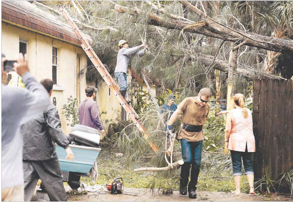
CHRIS URSD / Times Steve Miccio, 53, secures a limb with a rope as he and others work to remove a tree from the roof of his Gulf Road home Monday in Tarpon Springs. Miccio and his family weren't home when it fell.
