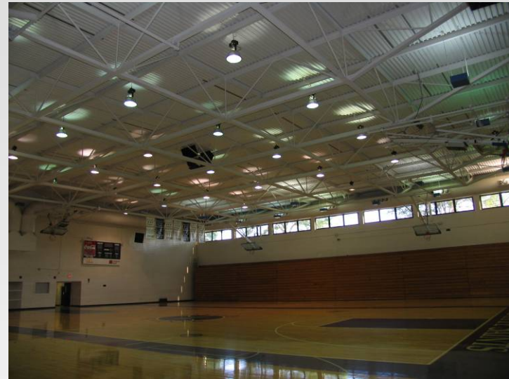
Before Energy Efficient Lighting
