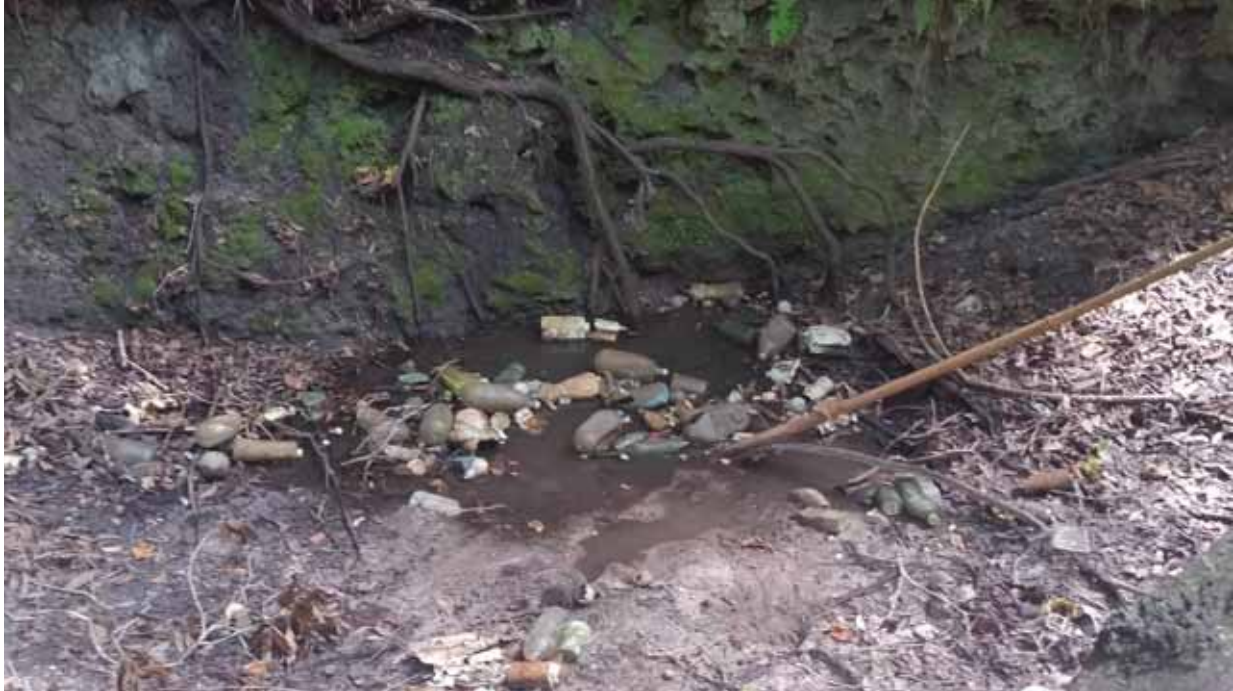
Figure 23. Standing water found in the bottom of one of the depression features.
