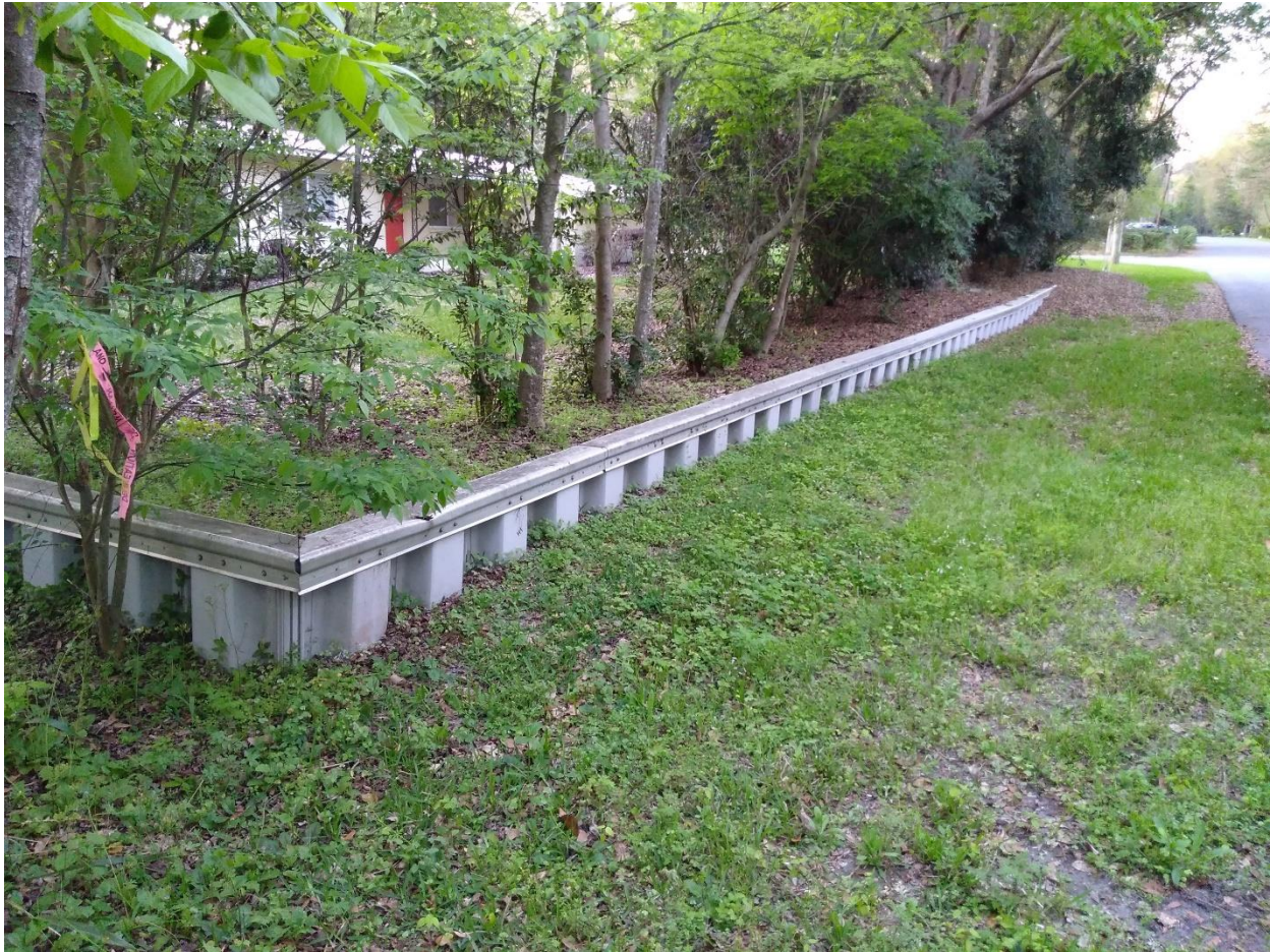
Photograph 3. Mason Manor floodwall, eastern terminus, facing north at the southern end of Northwest 25 th Terrace toward the intersection of Northwest 25 th Terrace and Northwest 10 th Avenue. Photograph by Wood in March 2018.
