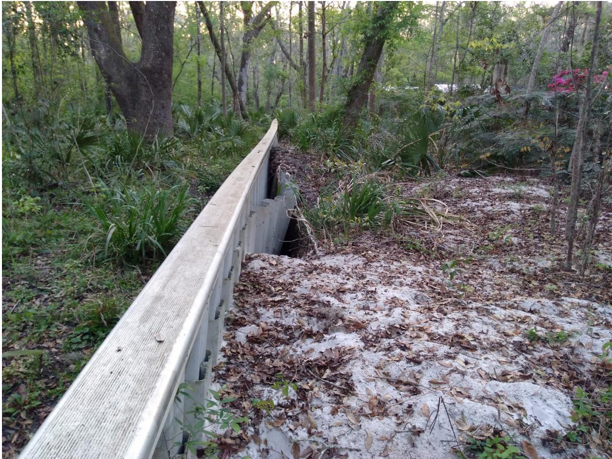
Photograph 6. Mason Manor floodwall, about 100 meters west of Northwest 25 th Terrace, facing west at an undermined part of the sheet pile wall. Hurricane Irma floodwater likely deposited white sand on the north side of the undermined section, in September 2017. Photograph by Wood in March 2018.
