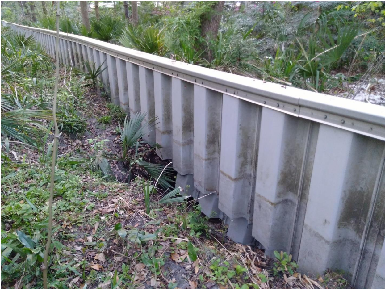
Photograph 5. Mason Manor floodwall, about 100 meters west of Northwest 25 th Terrace, facing northwest at an undermined part of the sheet pile wall. Hurricane Irma floodwater likely deposited white sand on the north side of the undermined section, in September 2017. Photograph by Wood in March 2018.
