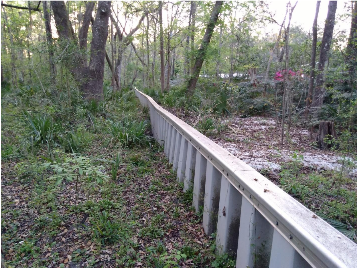
Photograph 4. Mason Manor floodwall, about 100 meters west of Northwest 25 th Terrace, facing west toward an undermined part of the sheet pile wall. Hurricane Irma floodwater likely deposited white sand on the north side of the undermined section, in September 2017. Photograph by Wood in March 2018.
