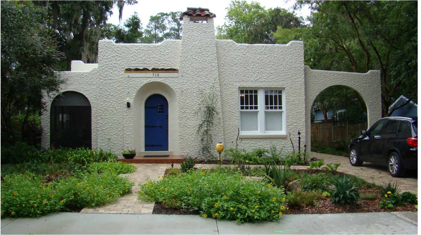
Front Elevation demonstrating new paint work, new porch stoop with tile, new walks and pavers at drive.
