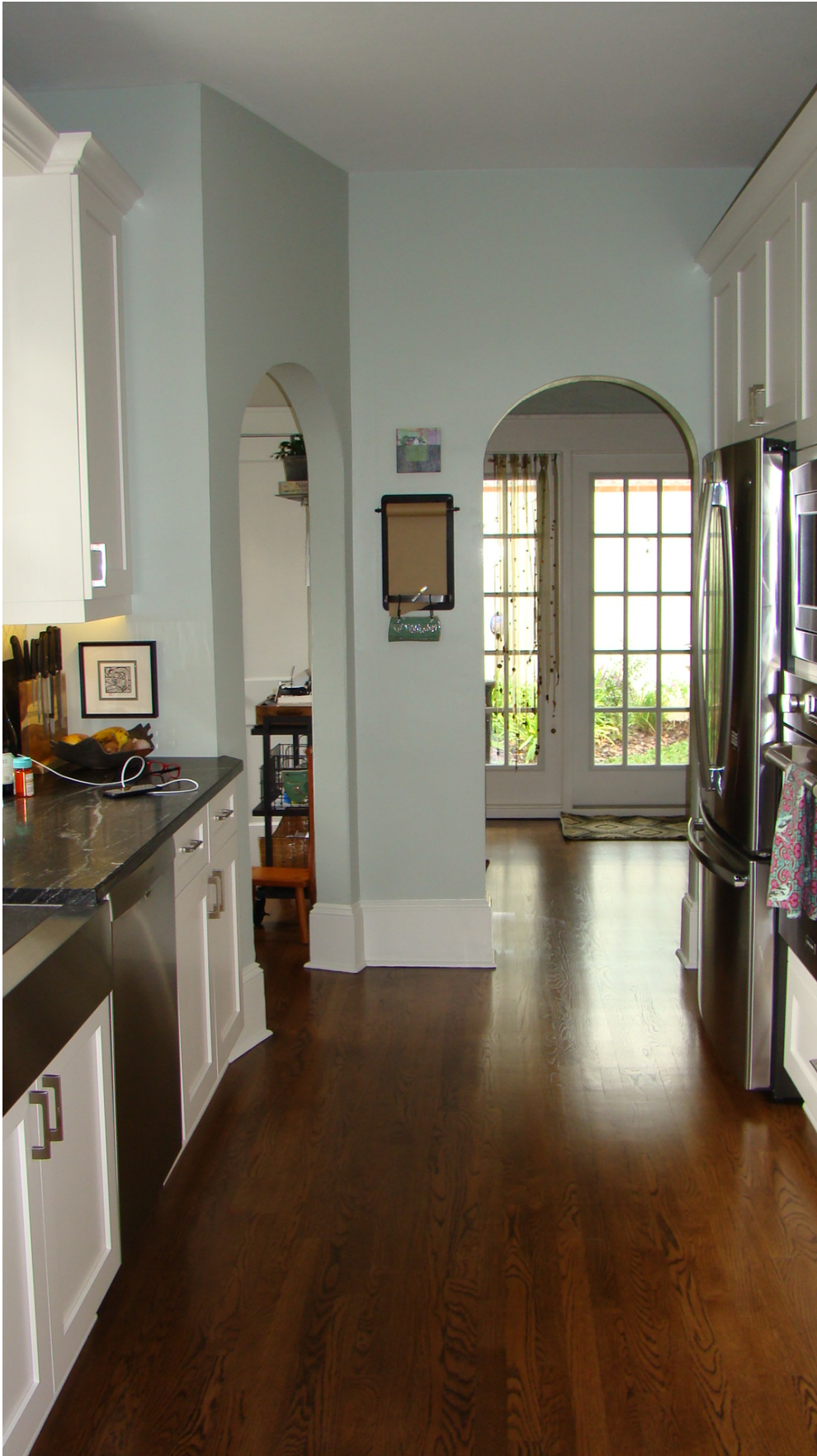
New Kitchen cabinets and counters, appliances and oak flooring to match the original. Original archways were maintained.
