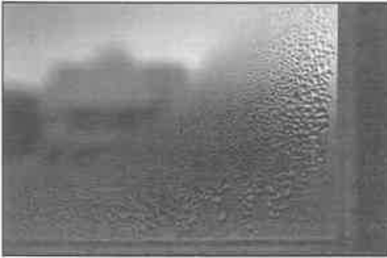
Condensation on the inside of a window-pane.
